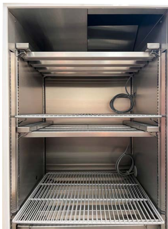
Shelf lights installed with power cables going through the 54 mm port holes.
