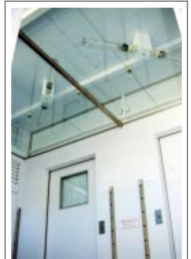
TPG-5000-TH INTERIOR AND LIGHT LOFT
